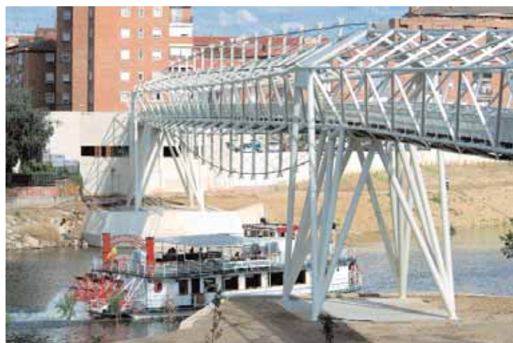
In addition to its mechanical function, the external prestressing cable grid looks like the fish baskets which inspired the architect's design.
