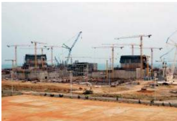
256 prestressing cables were installed in the two containment vaults in Kudankulam (India).
